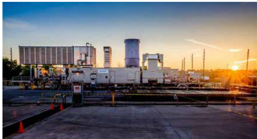
The fast power mobile gas turbine unit will provide up to 41 megawatts of power for approximately 200,000 homes in northern Afghanistan.
